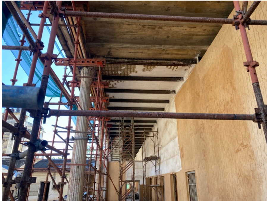
Figure 4: A deteriorated slab of a walkway in the House of Wonders exposing its only bottom reinforcements (Author).
